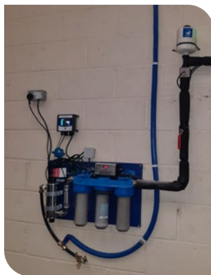
Image: Pipework from the 2,600-litre tank to the fine filtering system.
