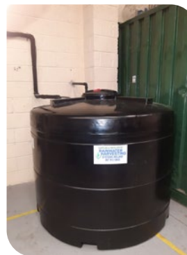
Image: Storage tank.
