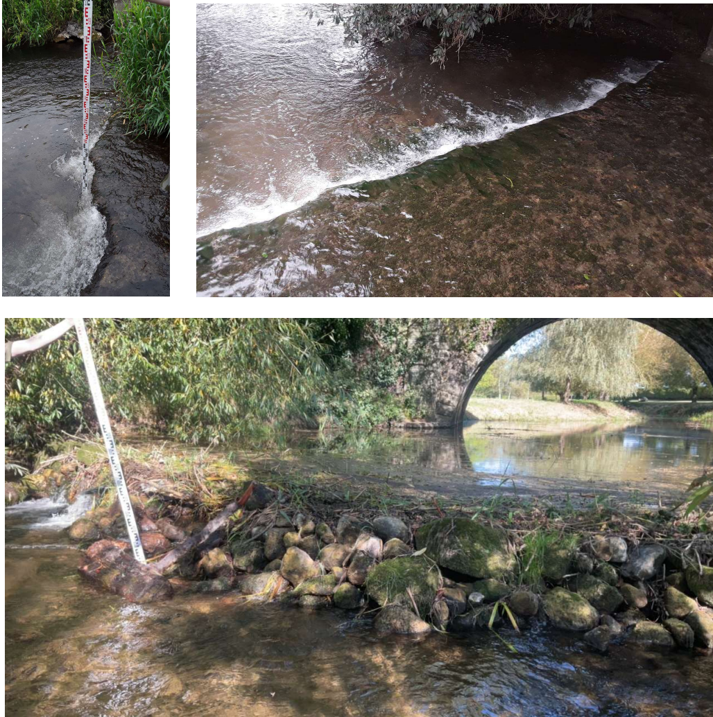
Figure 4.4 Top: Shallow bridge aprons posing both a jump and swim barrier to migratory species present on the Morningstar (C1/31) within 200m of each other (left: 24_792_26; right: 24_792_19). Bottom: stone weir present in the lower reaches of the channel.
