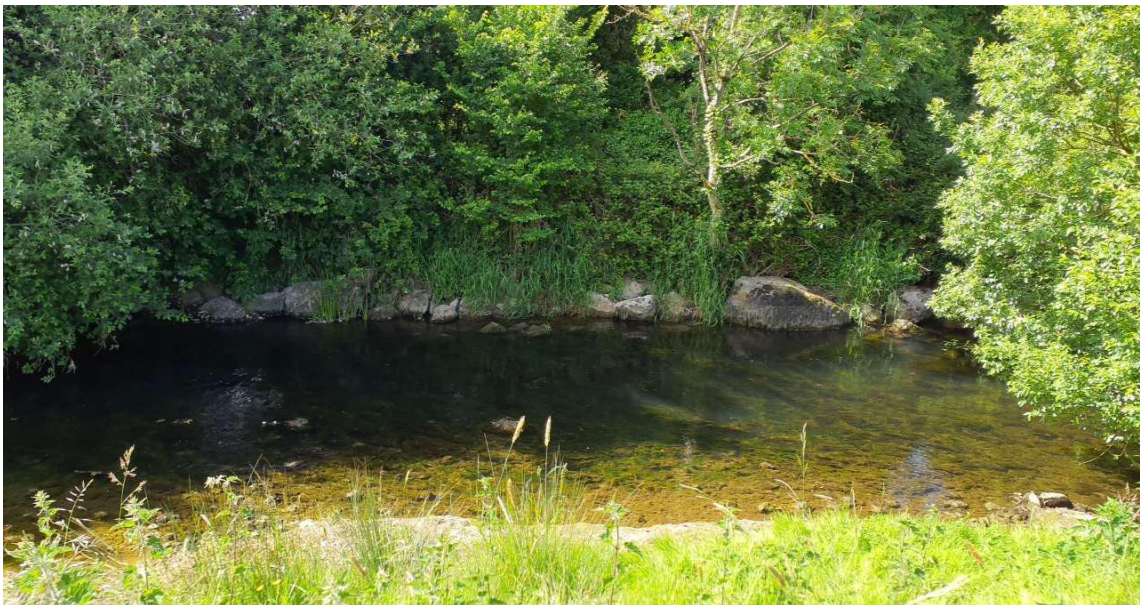
Figure 3.6 Site on the Camoge River (C1/25). Artificial deflectors have not naturalised since installation (top). Bank reinforcement evident on over-widened channel and algae is dominant in the instream area (bottom).
