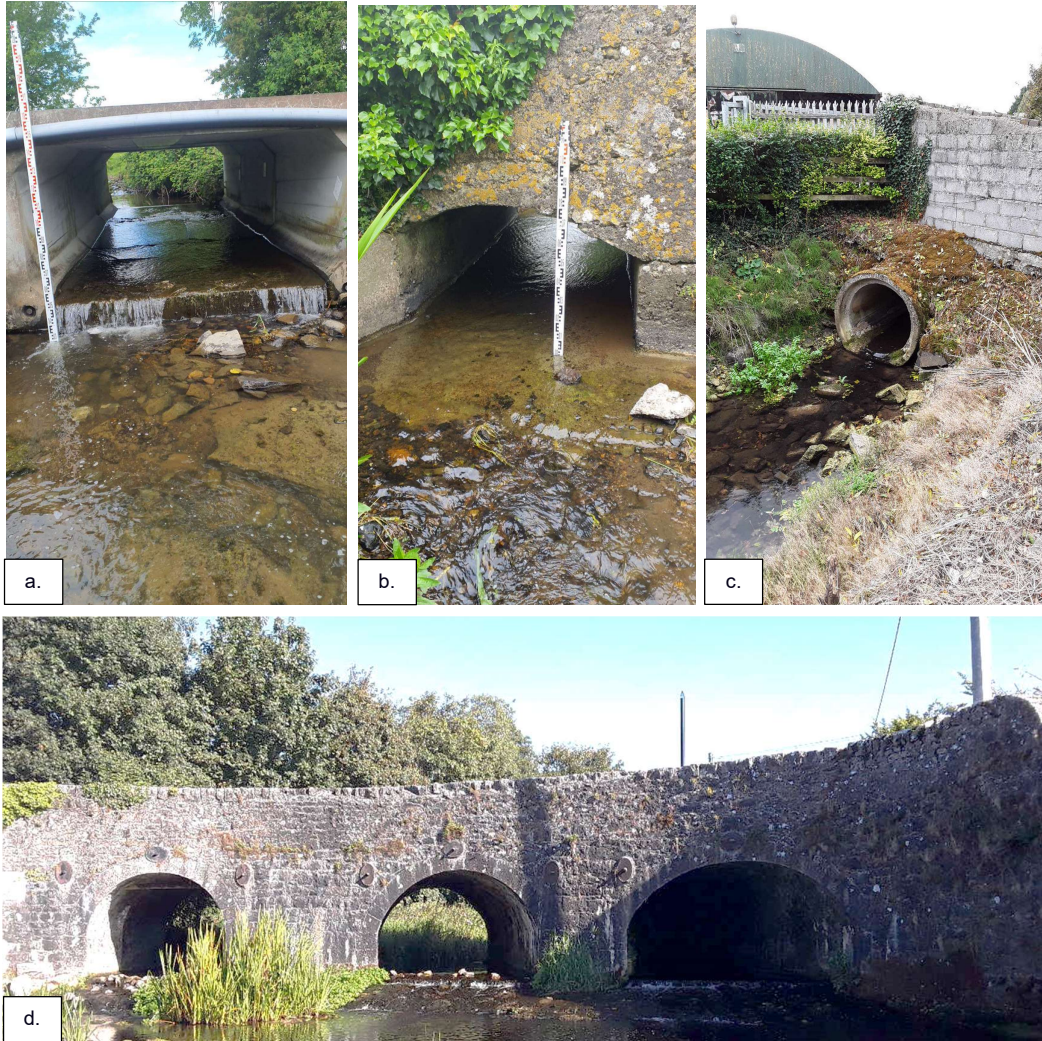
Figure 4.2 Examples of barriers classified as culvert / bridge apron. (a. 24_9_3; b. 24_9_6; c. 24_1688_46a; d. 24_795_76).
