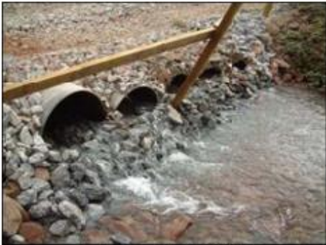
Temporary crossing impassable to fish life.
