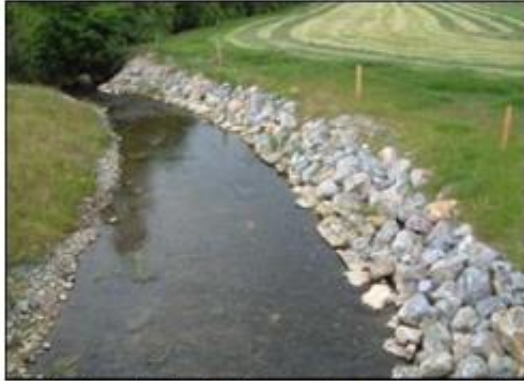
The boulders in these bank protection works are not large enough, not sunken below stream bed level and likely to be undercut and dislodged in a storm event.
