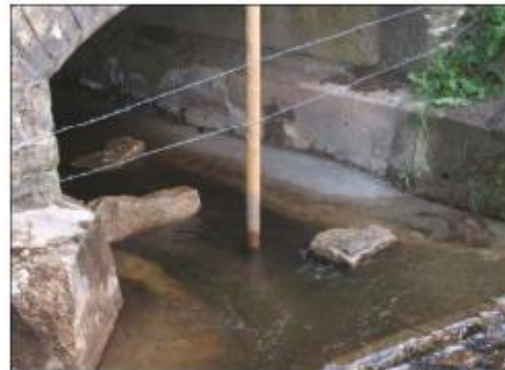
Large stone baffles held in position on concrete apron with stainless steel dowel rods drilled into both the apron and stones. (Poor placement of the livestock fencing as shown in the photograph has the potential to cause blockage by catching debris.)
