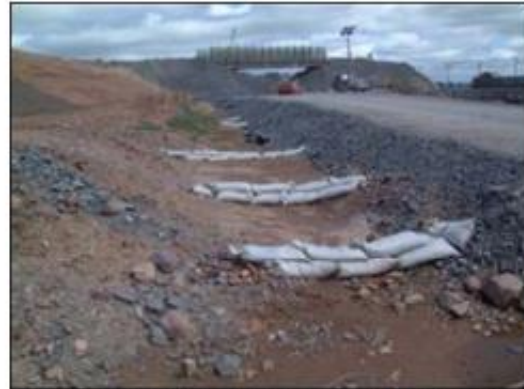
Silt discharge minimisation by providing retention areas to reduce discharge velocity and allow settlement during rainfall events.
