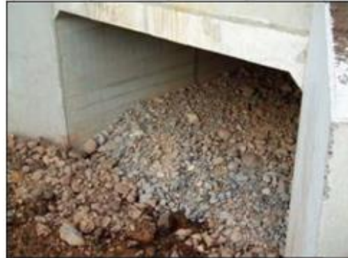
Off-line culvert at construction stage back filled with gravel. The size range and depth of fill required will be site specific.
