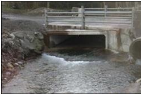
Box culvert positioned at incorrect level. Upstream fish passage is made difficult. Culvert invert should be 500 mm. below existing bed level and back filled with clean gravel to match the existing stream profile.
