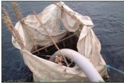
A screened abstraction point using terram fitted over a fabricated support frame.
