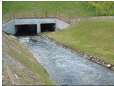
Looking from upstream towards a culvert arrangement. Moderate and flood flows are conveyed in the right hand culvert. Entry to that culvert is dictated by the invert and contour of the right hand portion of the newly created river channel. The left hand bank finished batter angle is approx. 45°. The first portion of the right hand bank to convey the moderate flow is battered to approx. 30°. The extreme right bank area is battered to approx. 45° to convey flood flows.
