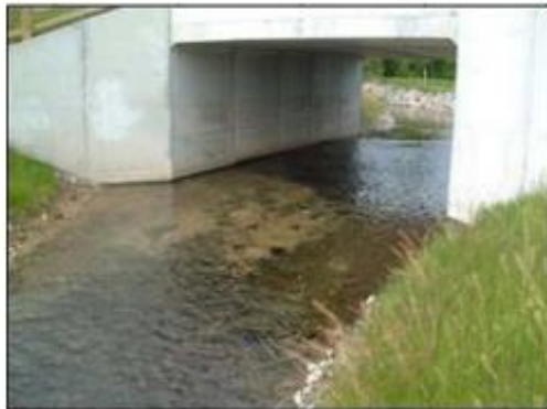
Excessively wide culverts can result in reduced current speed, ponding, and siltation of instream gravels.
