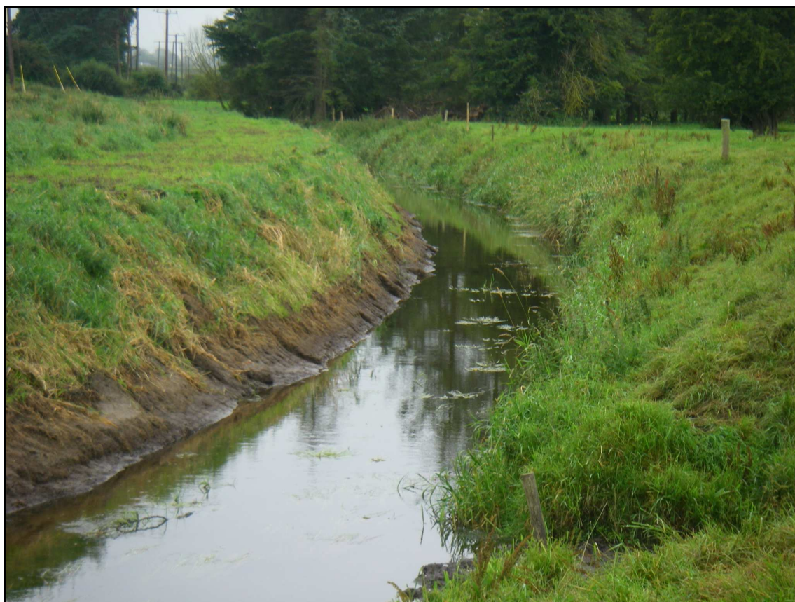
Plate 4.7. The River Boyne site at Boyne Bridge near Edenderry, Co. Offaly, surveyed shortly after maintenance work by OPW
